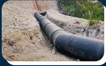
14.5MW Siguil Hydro Power Plant Maasim, Sarangani
